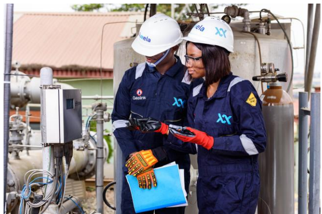
[Careful pipeline maintenance and management]
